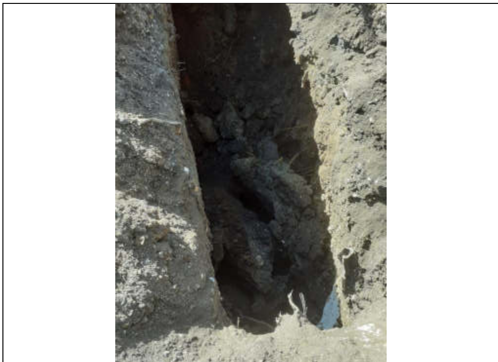
Plate 274: TP131 pit collapse.
