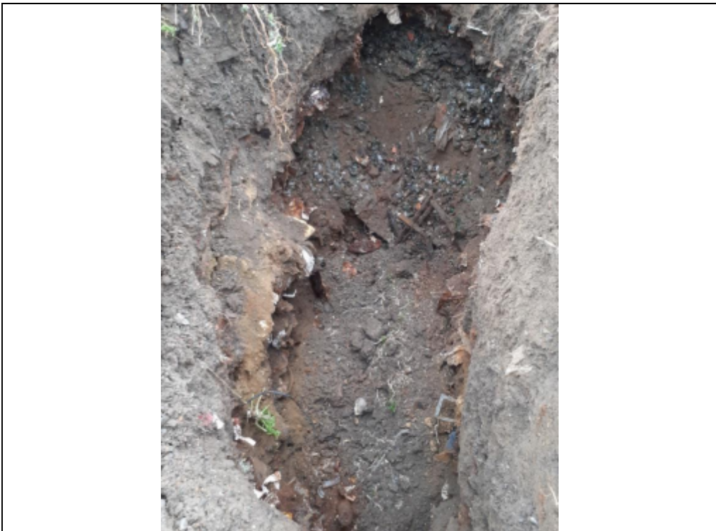
Plate 128: TP116 showing pit collapse.
